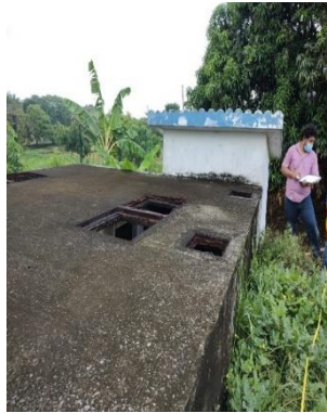
Figura 51. Digestor aerobio PTAR Paraíso-San Manuel.
